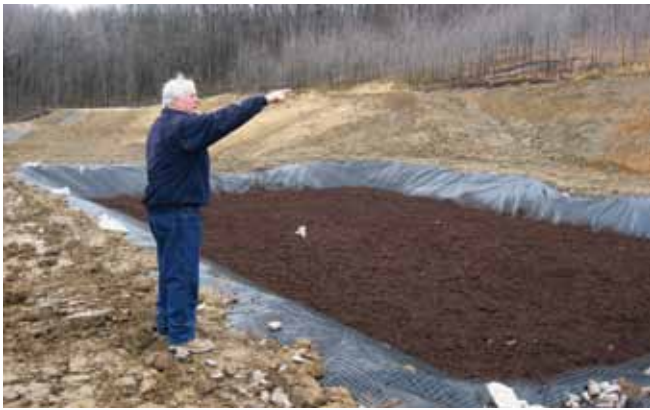
Pennsylvania Fish & Boat Commissioner Thomas Shetterly of the Chestnut Ridge Chapter of Trout Unlimited surveys the chapter's acid mine drainage treatment project on Morgan Run in Fayette County.
