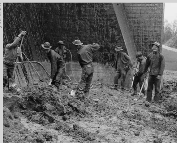
Members of a CCC crew work on the foundation of the dam that created Laurel Hill Lake at Laurel Hill State Park.
