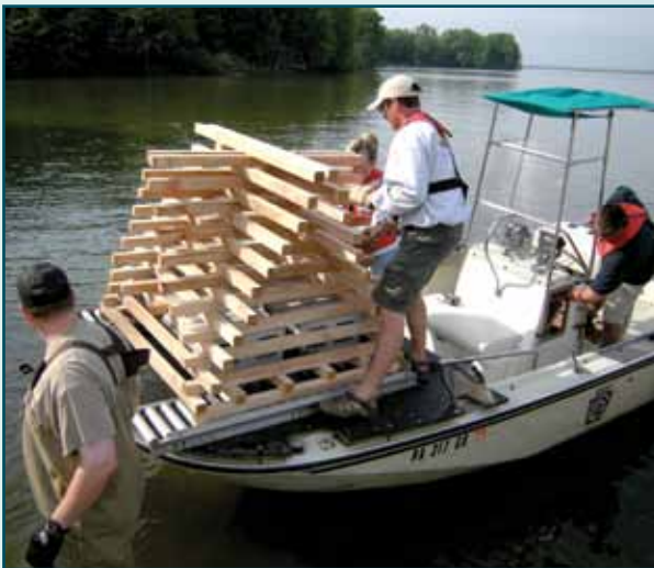
The rollers on crib boats make it easier to install porcupine cribs.
