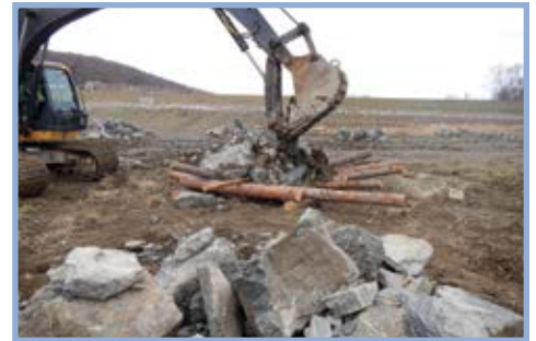
PFBC’s Division of Construction and Maintenance finishes a structure at Lake Nessmuk, Tioga County.
