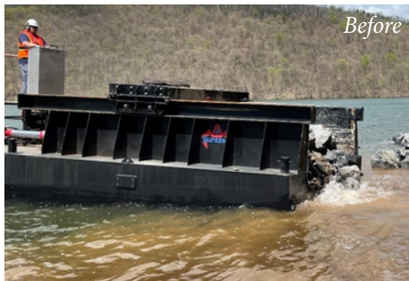
PFBC staff use a rock barge to place stone along an eroded shoreline at Raystown Lake, Huntingdon County.
