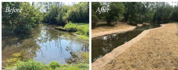
Buffalo Creek, Union County, before and after habitat improvement structures were installed.
