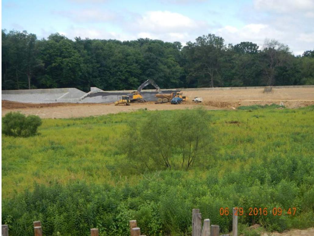
Repair of the dam and spillway at Glade Run Lake in 2016 is now complete and the Lake is recently refilled.
