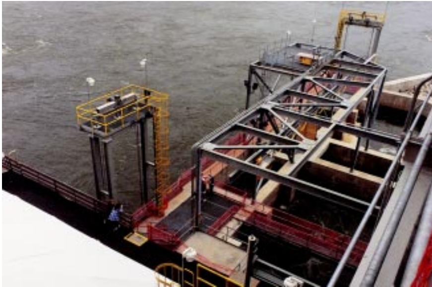
The new fish lift at Safe Harbor Dam began operation in 1997. This fish lift, like Conowingo Dam's east lift, passes migrating fish directly into the pool above the dam.
